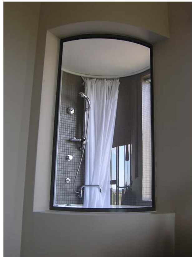
6mm clear toughened curved glass shower enclosure Balgownie Resort, Varra Valley Victoria
